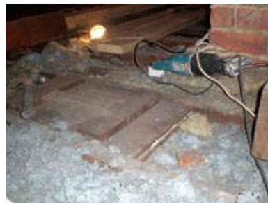
Figure 6 Loose asbestos used as loft insulation
