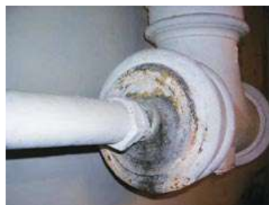
Figure 30 Amosite and chrysotile packing on waste pipes
