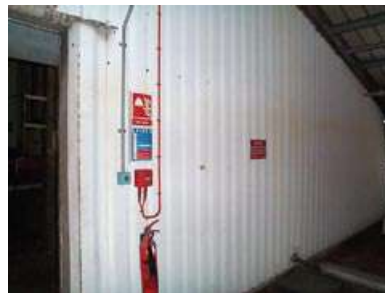
Figure 38 Chrysotile/bitumen coating under metal cladding
