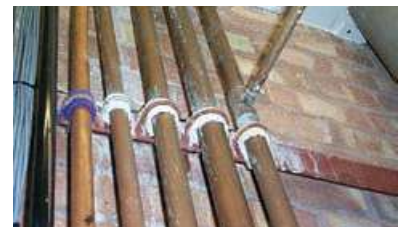
Figure 29 Chrysotile cloth on pipes
