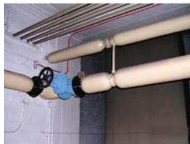
Figure 4 Pipe uncertainty: Top pipe is non-asbestos. All pipes should be sampled
