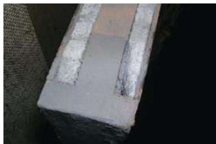
Figure 14 Asbestos panels inside fire door
