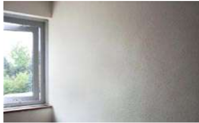
Figure 37 Asbestos textured coating on wall
