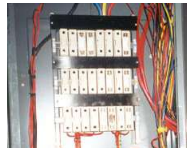
Figure 46 Asbestos tape flash guards in a fuse box
