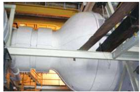
Figure 51 Vessel clad in amosite insulation
