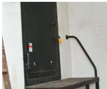
Figure 45 'Durasteel' composite steel and asbestos fire door
