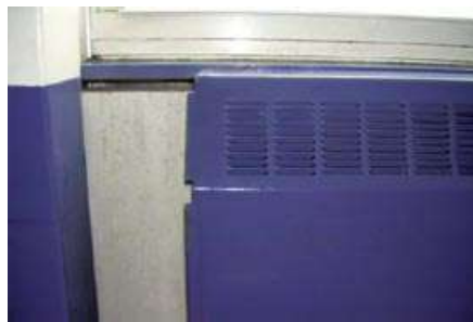
Figure 50 Open electrical switchboard with asbestos flash guards
