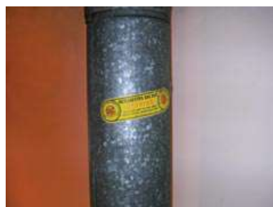
Figure 43 Metal clad gas flue containing chrysotile lining
