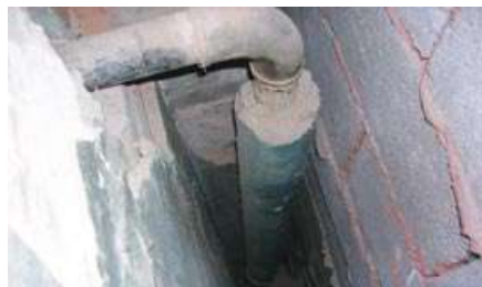
Figure 9 Lagged pipe in wall cavity
