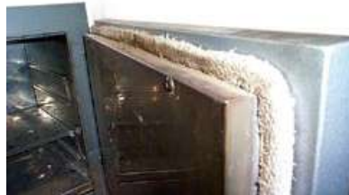
Figure 26 Asbestos rope seal on drying oven
