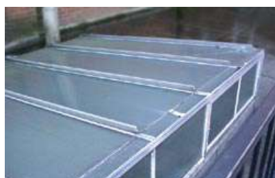
Figure 31 Chrysotile string on skylights
