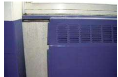
Figure 19 AIB behind school radiator unit
