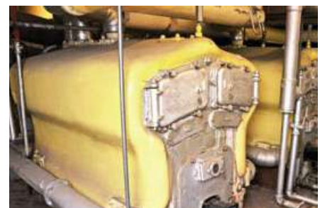
Figure 13 Amosite lagged boiler with hard plastic coating
