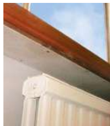
Figure 20 AIB panel between radiator and window
