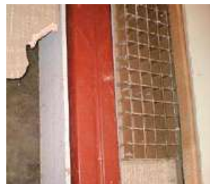
Figure 21 AIB column fire protection in CLASP building
