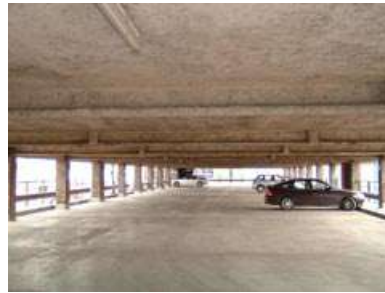
Figure 7 Sprayed limpet on car park roof
