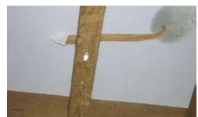
Figure 25 Chrysotile paper on strawboard ceiling panels
