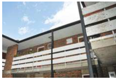
Figure 18 AIB exterior panel on open walkway
