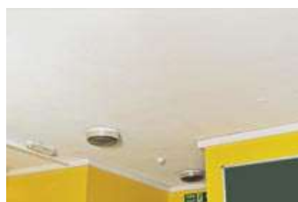
Figure 36 Asbestos textured coating on ceiling
