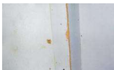
Figure 24 Chrysotile paper on fibreboard boxing
