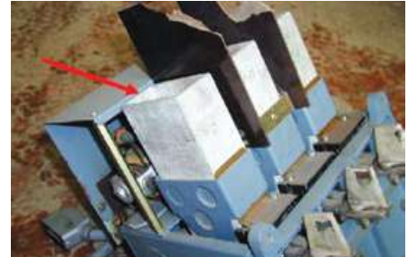
Figure 49 Electrical switchgear with asbestos flash protection
