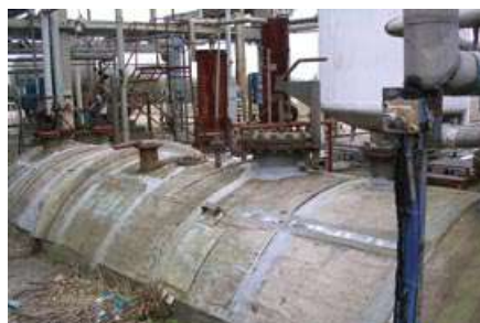
Figure 12 Lagging on large petrochemical vessel
