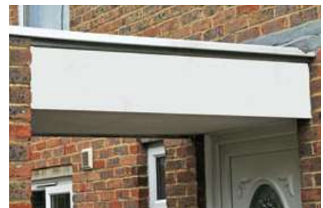
Figure 15 AIB panel in porch
