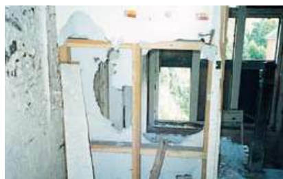
Figure 7 Asbestos insulating board wall panels badly damaged
