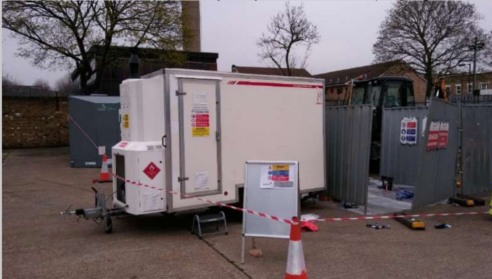
Photograph of site set-up (courtesy of Hydrock Consultants), signage, barriers and DCU:
