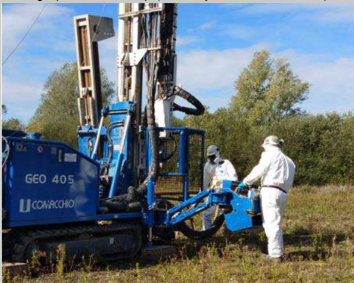
Photograph of site set up (courtesy of S M Associates), rotary drilling rig and operatives in PPE and RPE:
